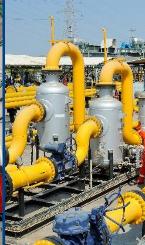
Natural Gas Skid
