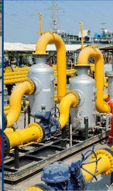
Natural Gas Skid
