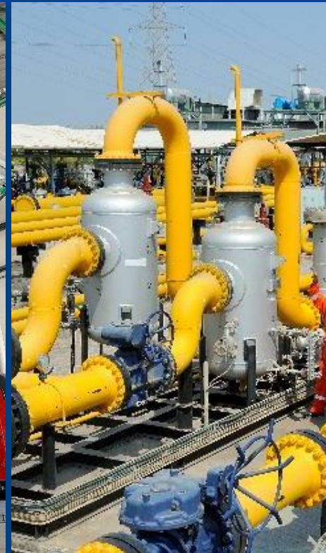
Natural Gas Skid
